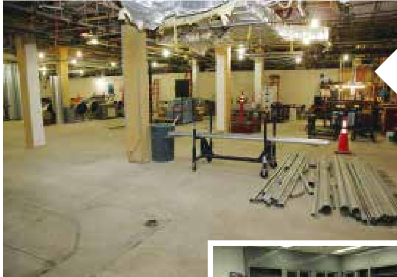
PROGRESS BEING MADE ON THE NEW PRECLINICAL SIMULATION FACILITY, FROM EARLY STAGE BELOW.
